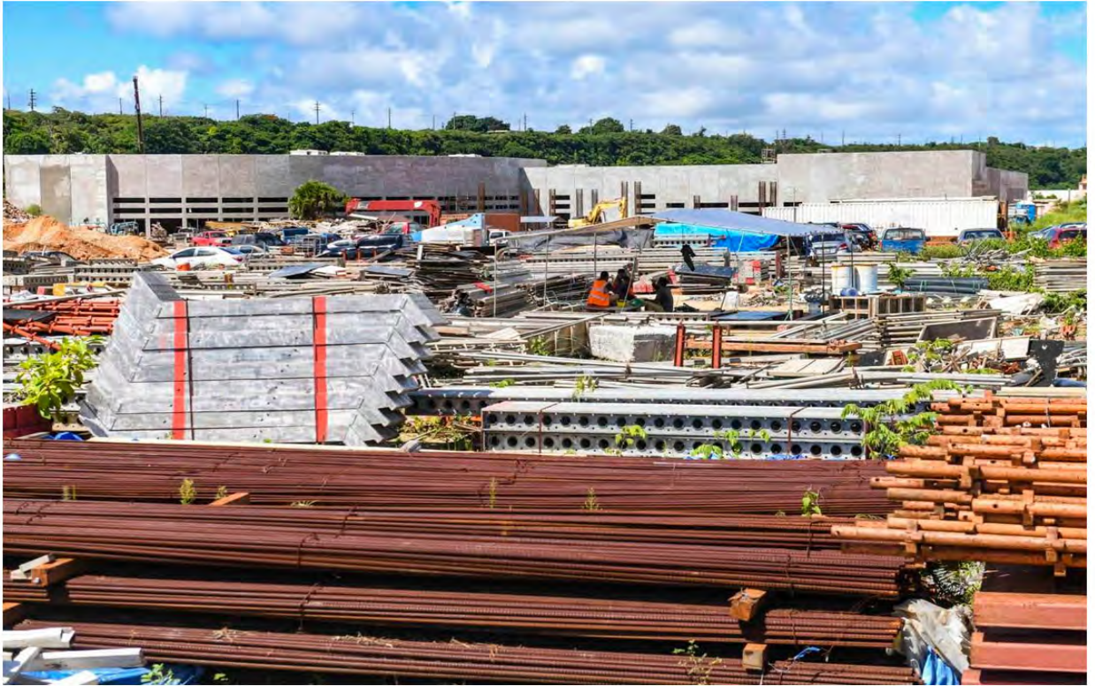
A trio of workers take time for a meal break under the shade of a canopy with the construction site of the Don Don Donki retail outlet on the corner of Marine Corps Drive and Chalan Pasaheru, or Route 10A, in Tamuning Aug. 18, 2022.
