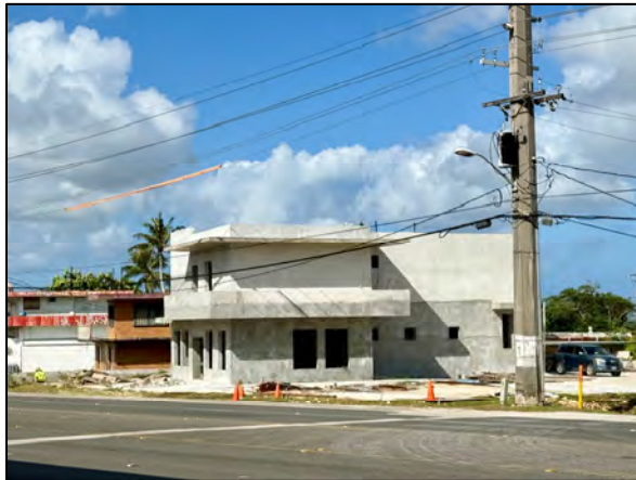
A half-finished two-story building sits on the old Oriental Kitchen restaurant property, with construction ongoing, almost three years after an explosion destroyed the restaurant.
