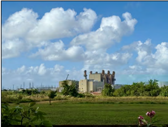
The Ukudu Combined Cycle Combustion Turbine Power Plant nears completion in Dededo, with September 2025 as the target.
